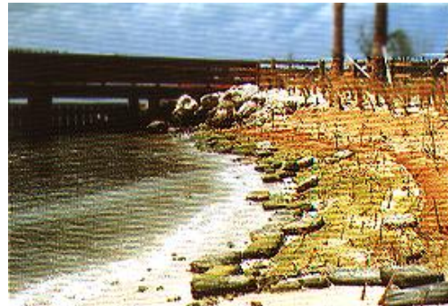
GEOCOIR®/DeKoWe® 700 being used in a vegetated geogrid and blanket application to protect a sand embankment from tidal and pleasure boat wave action.
